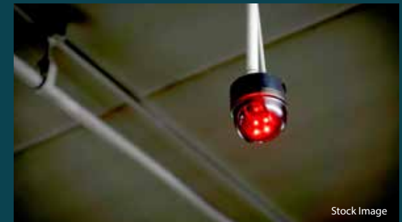
Energy Saving Sensor's Light In All Floor Lobby
