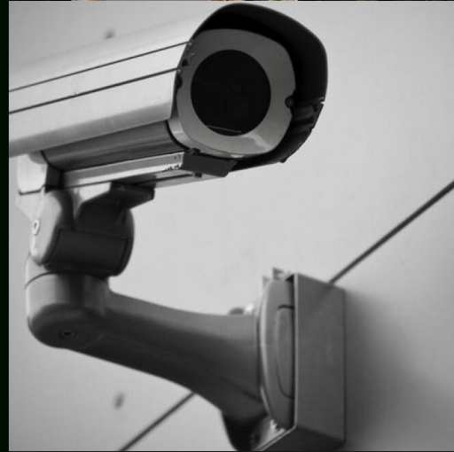
24x7 CCTV surveillance
