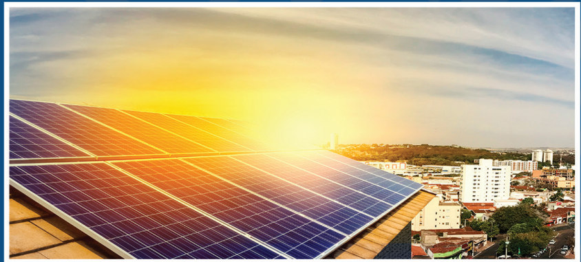
STP & SOLAR POWER
